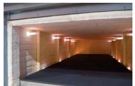
Furnace chamber with eight high-speed burners
