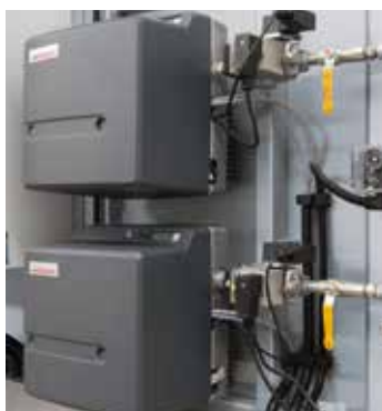
Gas burners for furnace heating and thermal post combustion
