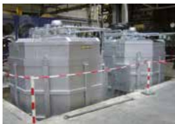
Forced convection pit-type furnaces SAH 5600/75 S in production
